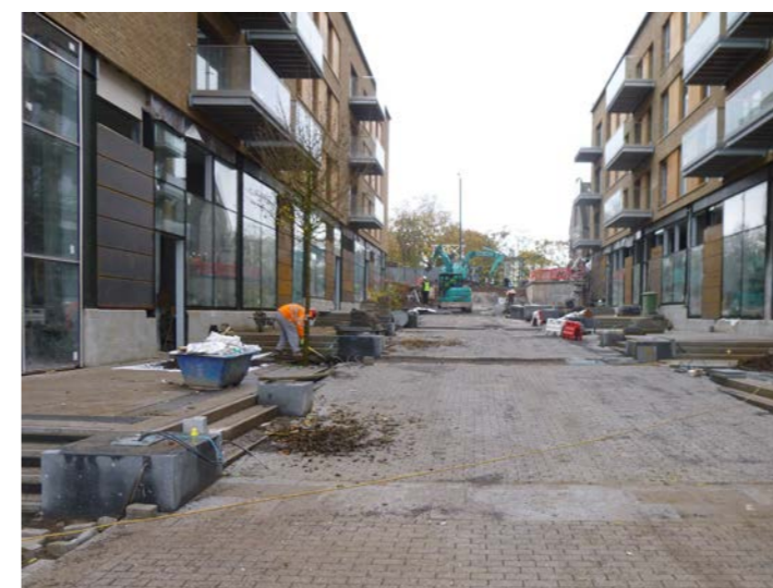
Wapping Wharf, Harbourside, Bristol - a local exemplar demonstrating a coherent spatial arrangement with active ground level uses, regular front doors, and overlooking balconies (under construction)
